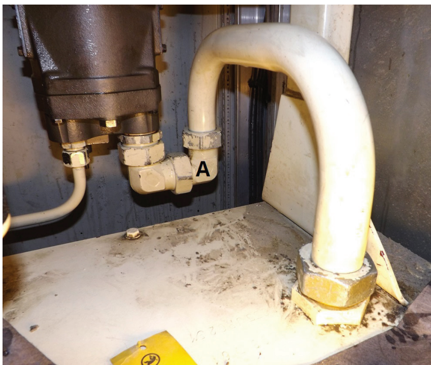
A fitting (marked "A") on this hydraulic pump suction line vibrated loose after 12 years, leading to aeration.
