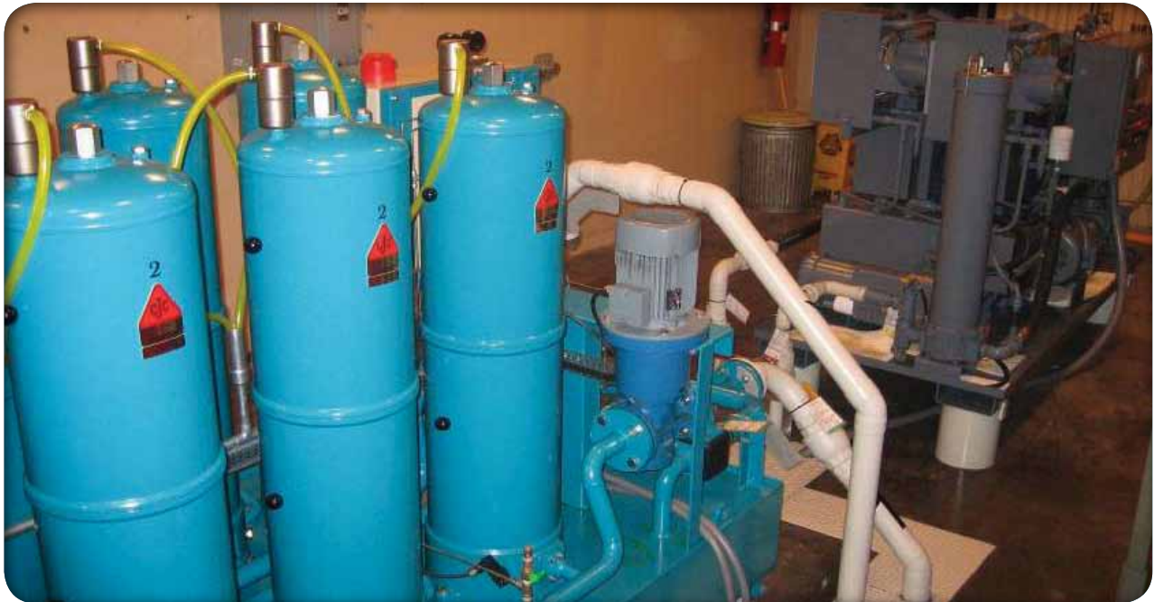
A vacuum dehydrator and filter system work to eliminate moisture, oxygen, and gases from transformer oil in Chief Joseph's oil room.
