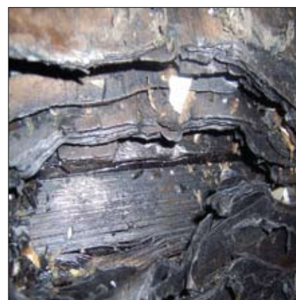
Fig. 11: Uncorrected thermal fault.
