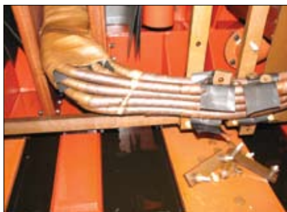
Fig. 2: Blue phase tapping leads and broken cleats.
