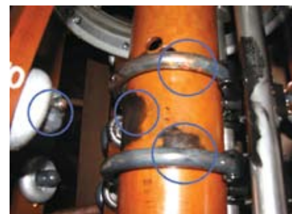
Fig. 3: Flash marks on fixed contacts and collector rings.
