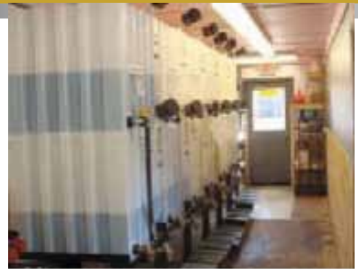
Polyethylene bulk tanks
