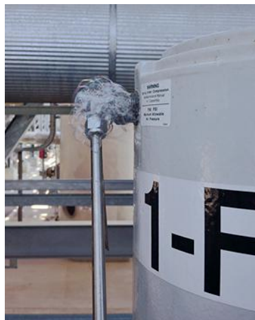
This view shows bubbles forming at a suspected leak site. The relatively large size of the bubbles indicates a substantial leak at low pressure.
