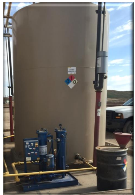
Kidney-Loop Filtration On Bulk Lube Oil Tank
