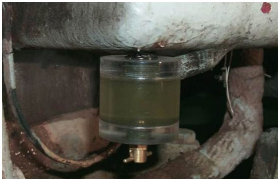
Figure 3. Oil sight glasses and other visual oil analysis products allow for constant monitoring of what's happening inside equipment.
