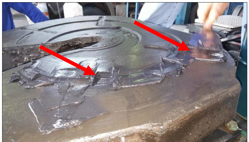
Use the scraper to fill the grease grooves on the top plate grease
